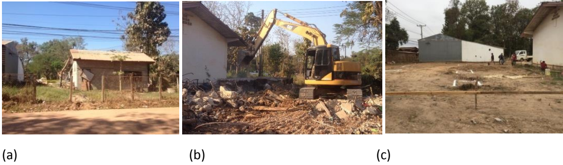
Figure 8. Demolishing old security guard house (a & b) and levelling the construction site (c)
