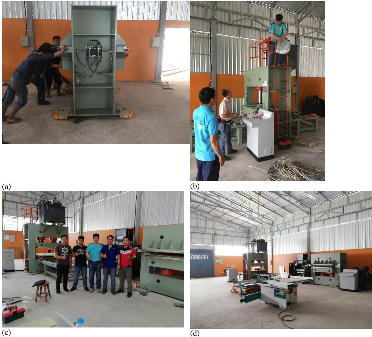
Figure 13. Installation and commissioning of machinery: moving into place using skates (a), electrical and hydraulic connection (b), NUoL staff receive training from BSY engineer (c), final installation (d).
