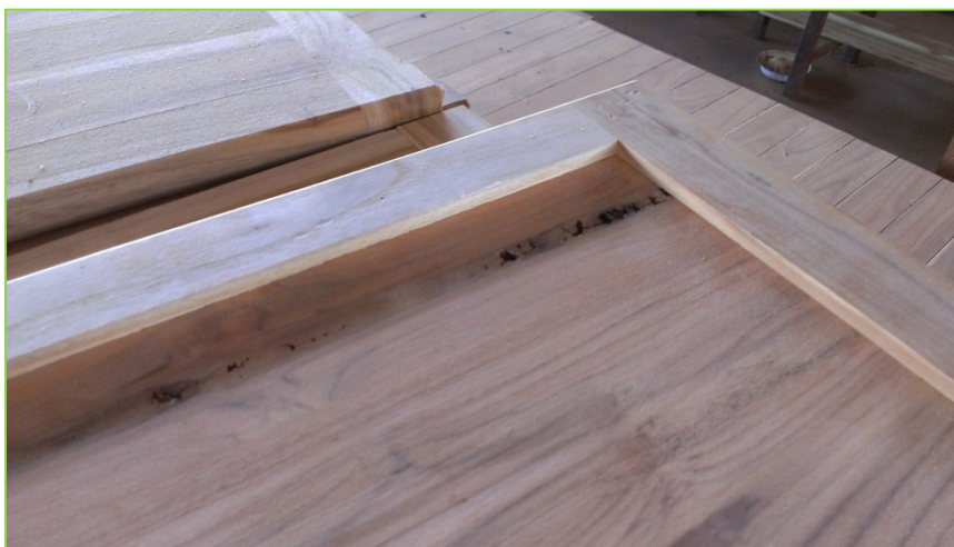
Figure 9 Finished panels where one strip is out of spec because of decay.
