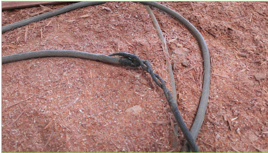
Figure 17 Damaged electrical wires in contact with wood dust is a potential fire hazard.
