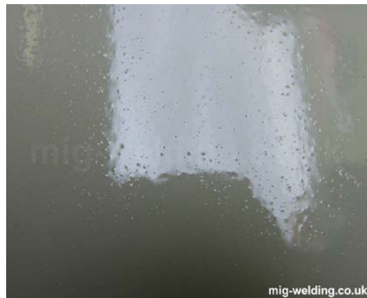
Figure 21: Overspray of finished surface (reproduced from http://www.mig-welding.co.uk/paint-faults/overspray.jpg )
